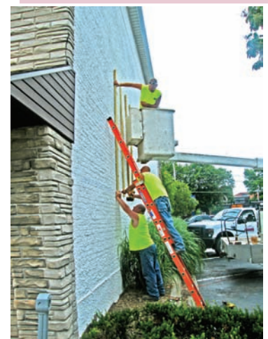
Morrison Public Works Employees Matt Lancaster, Drew Blean, and Mike Garland install mural framework.
